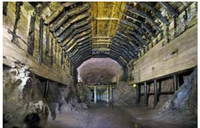
Impressive original shuttering still in place at Osowka. Beyond can be seen the remains of construction activity to excavate the pilot tunnel to full height. Photo Chris Rayner
